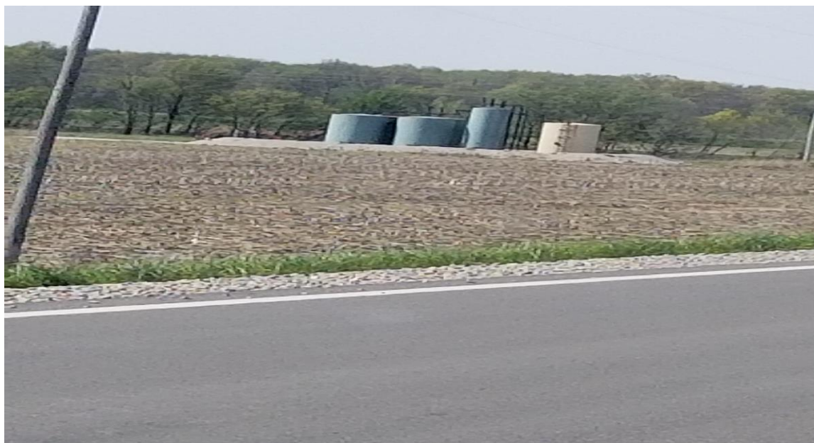
Figure 19.0. Typical Storage tanks for Pump Jack
