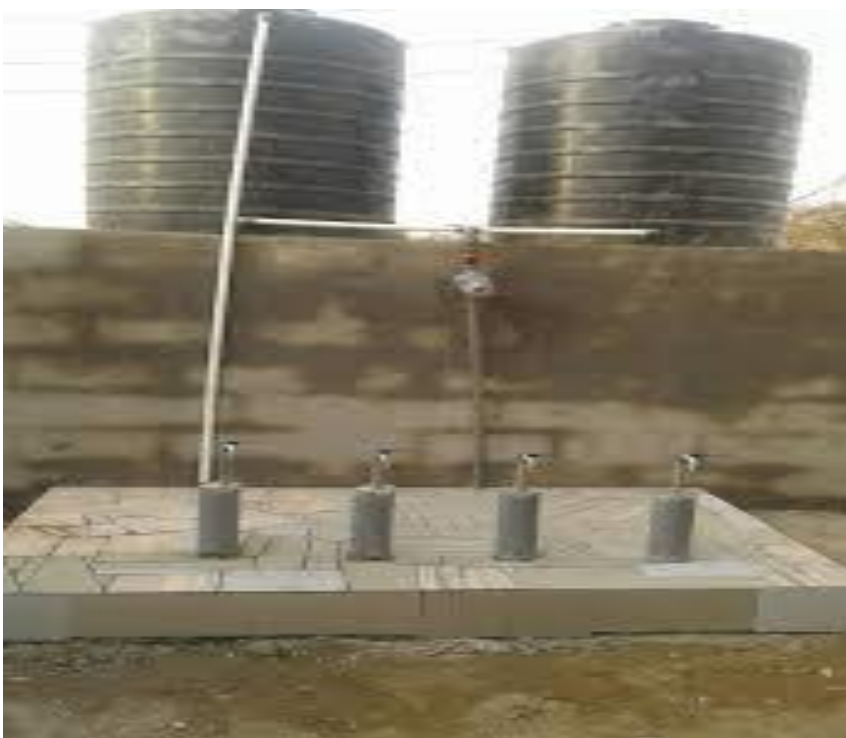
Figure 5. Picture of a private borehole.
